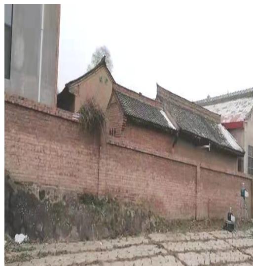
项目厂界设置挡墙
